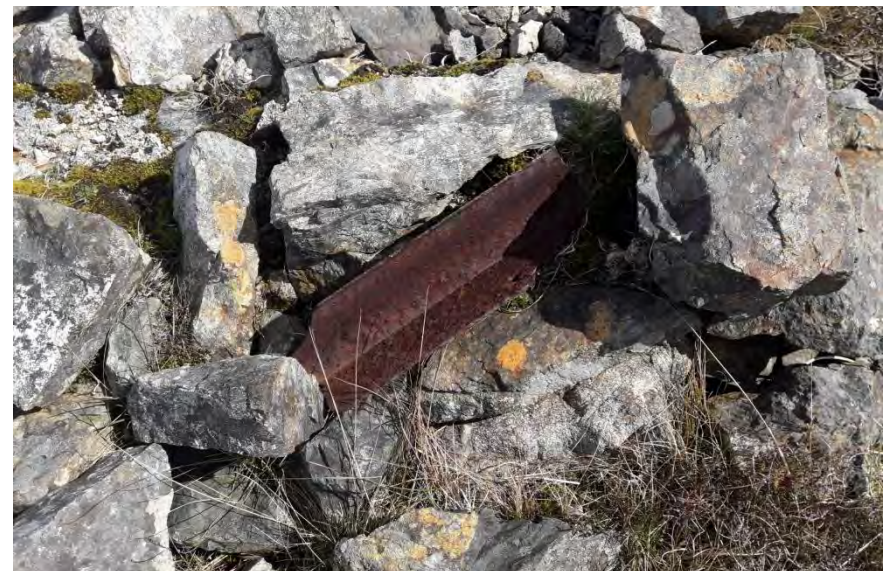
BNC 2: section of broken cast iron ogee gutter near E corner of building
