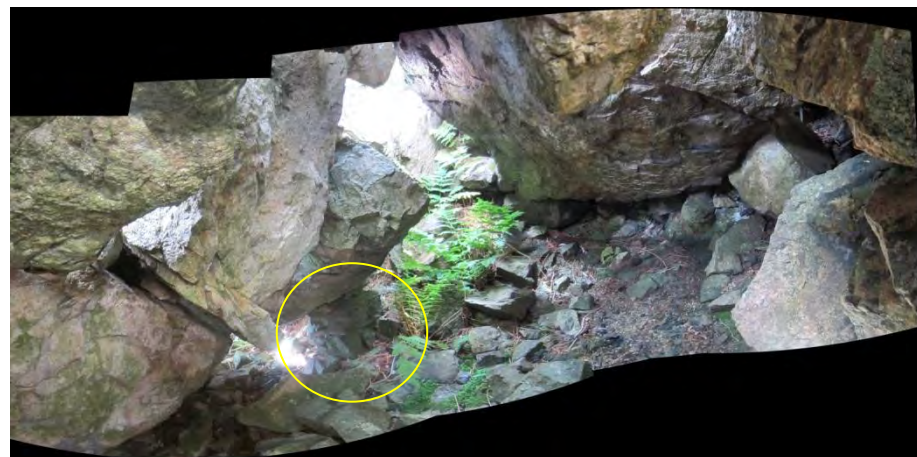
RB 7A: interior view looking SW with the drystone support pier highlighted
